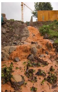
Erosion (source DE)
